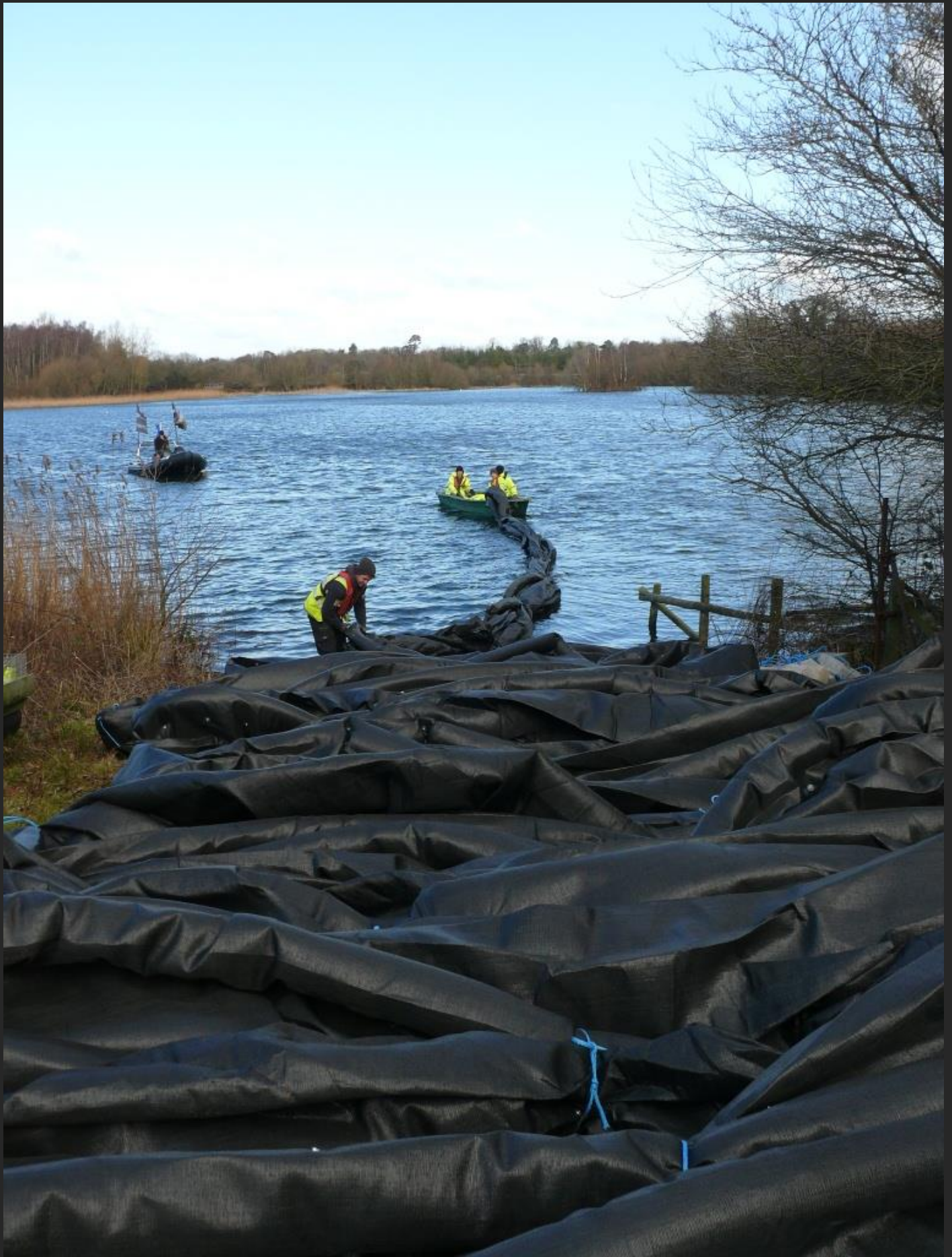
Once the netting team had cleared the area of fish the 160m fish exclusion curtain was floated into place, the dive team were on standby ready to deploy the anchors required to hold it where deployed for the period of the trial which could be several years.
